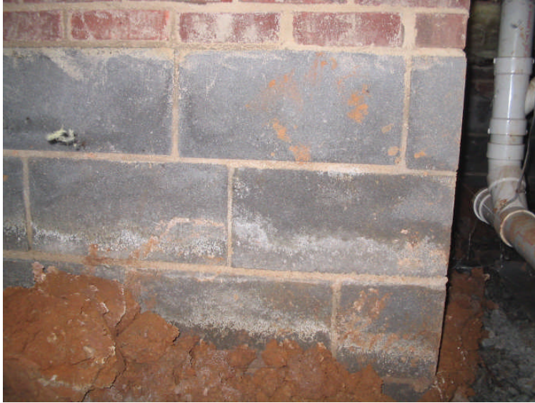
Efflorescence (white stains) on foundation wall.
